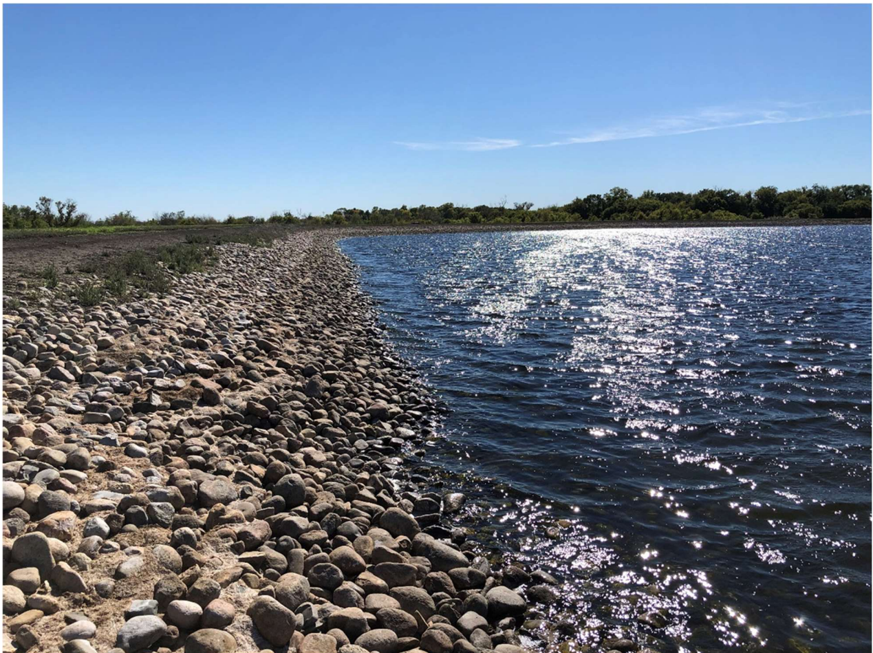
Figure 12. Drought Conditions Have Lowered the Water Levels at Hillsboro
