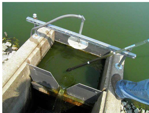
Figure 4. Algae and sludge Can Both Leave the Pond System to Affect BOD
